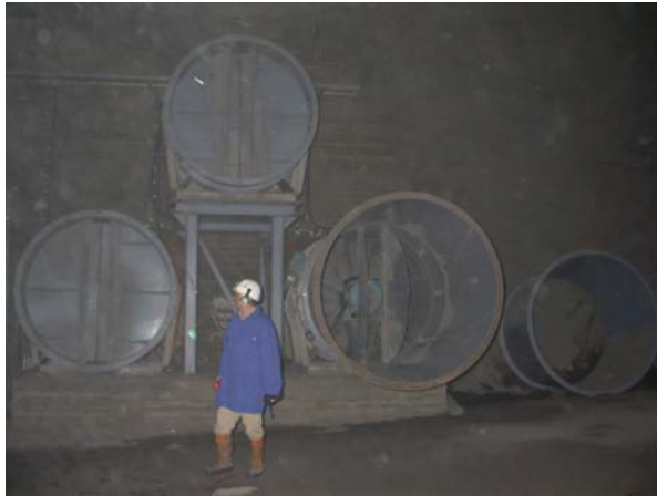
Figure 4. Extraction station (primary system)
