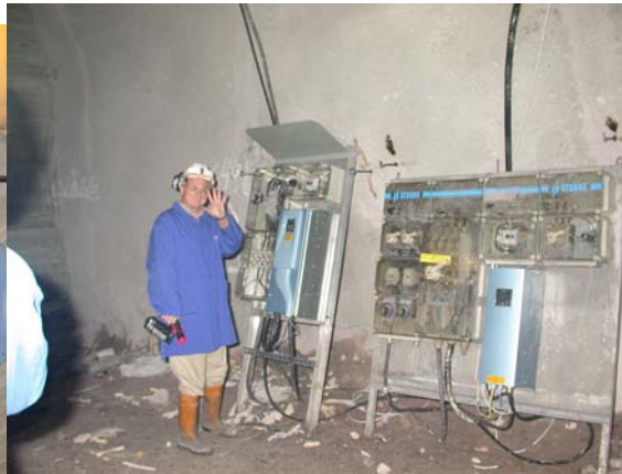
Figure 10. Fan control units with frequency inverters.
