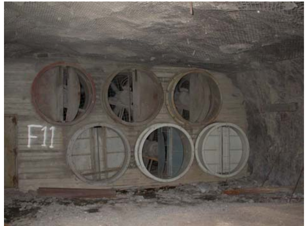
Figure 5. Fresh air ventilation wall (primary system)
