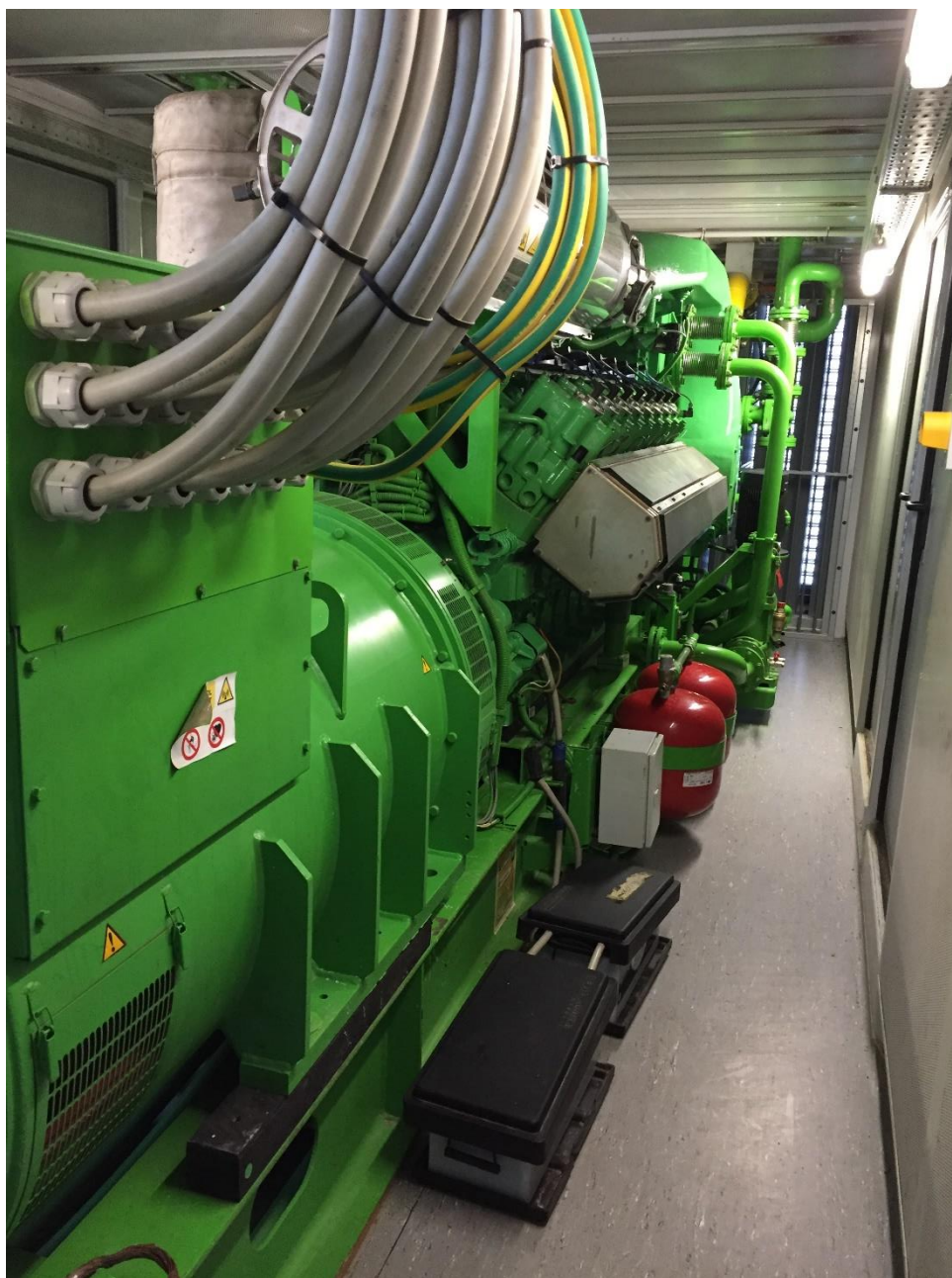
Image 4: Gas engine and electrical generator set group 2
