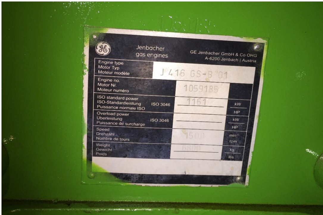
Image 3: Gas engine nameplate
