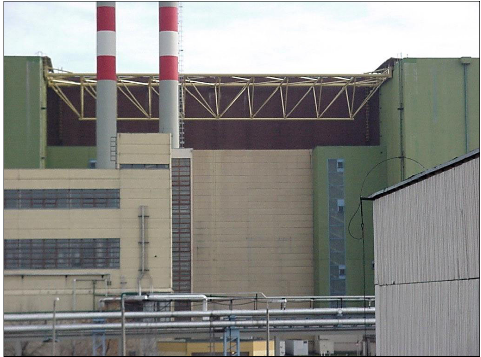
Figure 3-1: Bridge structure between the bubble towers for reinforcing the reactor building structures (PAKS 2012)
