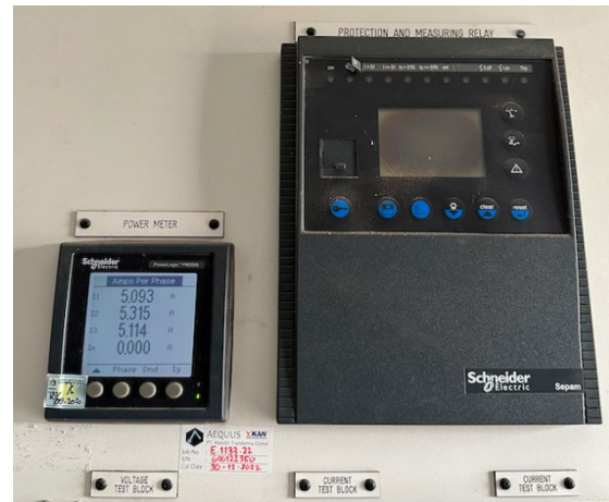
The energy meter (Schneider PM5560 0.2S)
