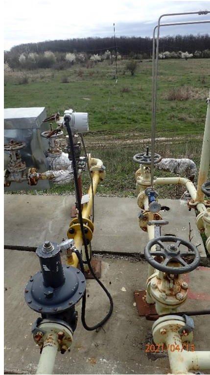
Figure C: Flare pipeline and flare stack
