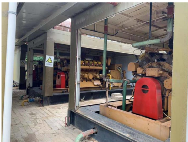
Image 3: The gas-fired generators
