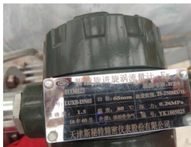
Image 6: The Vortex Flowmeter at point D
