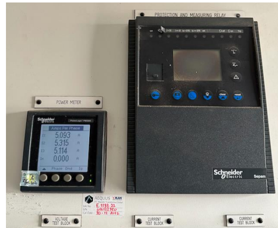
The energy meter (Schneider PM5560 0.2S)
